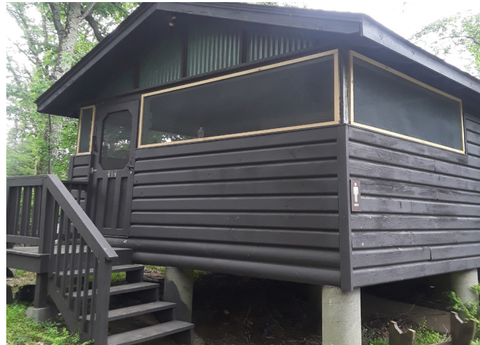
Harriman State Park Cabin. Building repairs and campground improvements of the Top of The Pines cabins (OPRHP).
