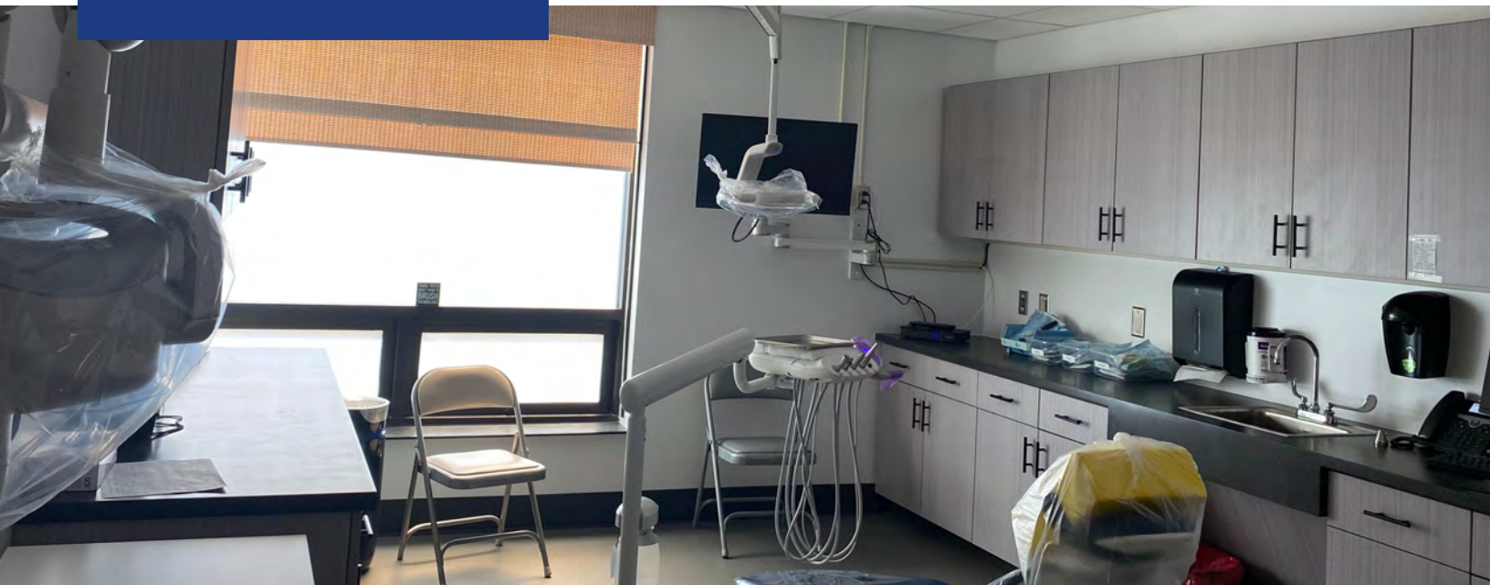
OPWDD, Broome DDSO, Renovation of Pod A into a Dental Suite, Binghamton
