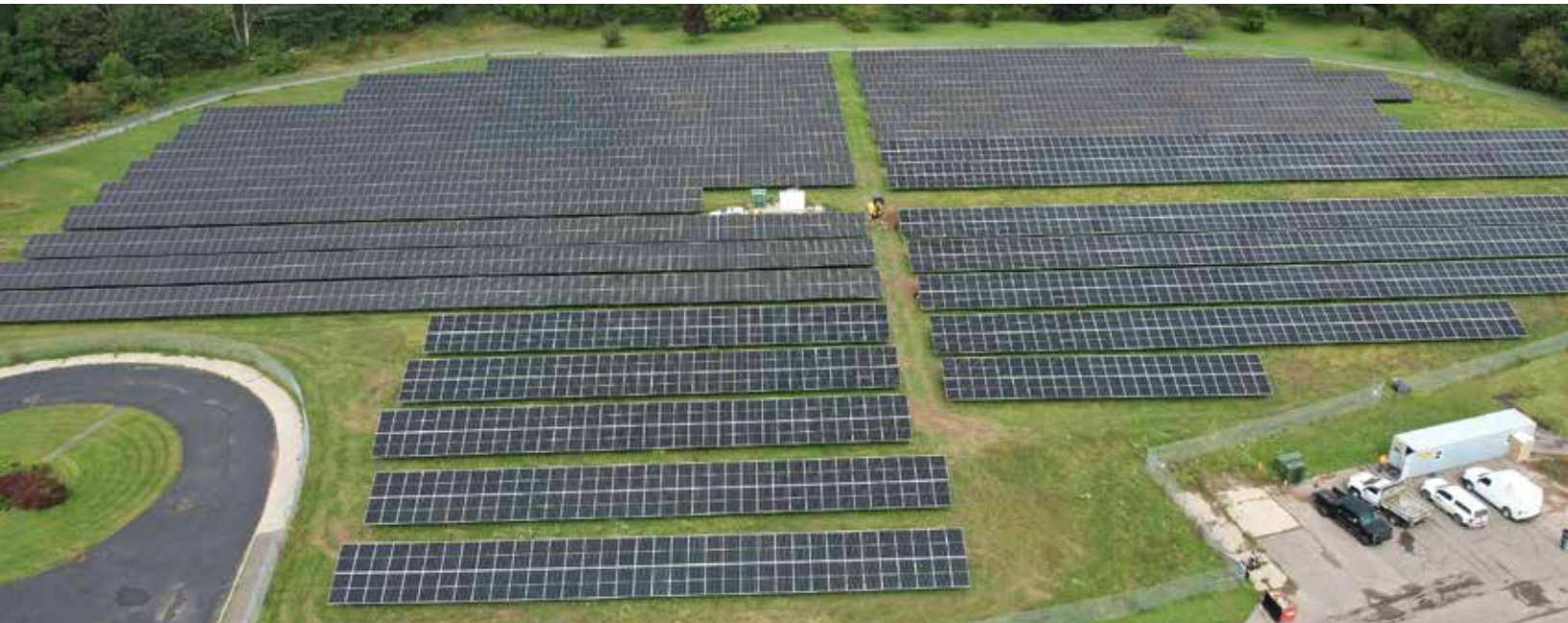
DASNY provided professional services to add solar array for NYS Veterans’ Home in Oxford, NY
