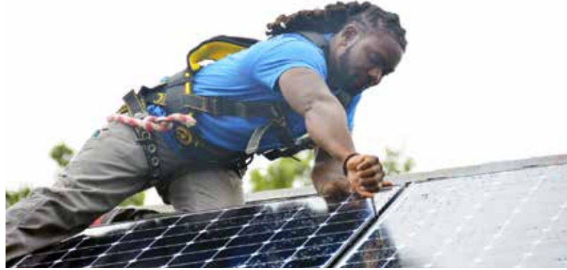
United Way of Long Island received a CCAP grant for their 'Net Zero Energy Challenge' to provide essential skills training for populations in need while transforming their headquarters with one of the largest solar arrays of any not-for-profit building in New York
