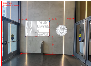
Existing Signage (MEC will provide it to the Vendor for installation) See added Photo #9
