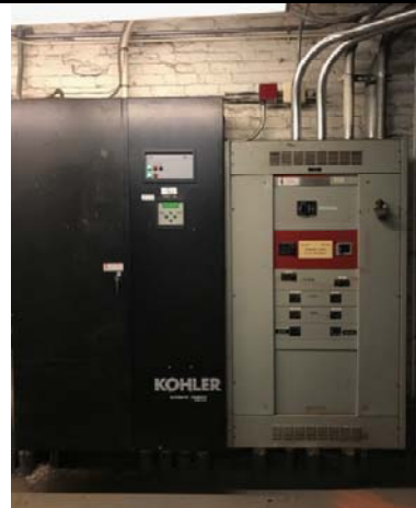
Photo E2- ATS & Emergency Distribution Board
