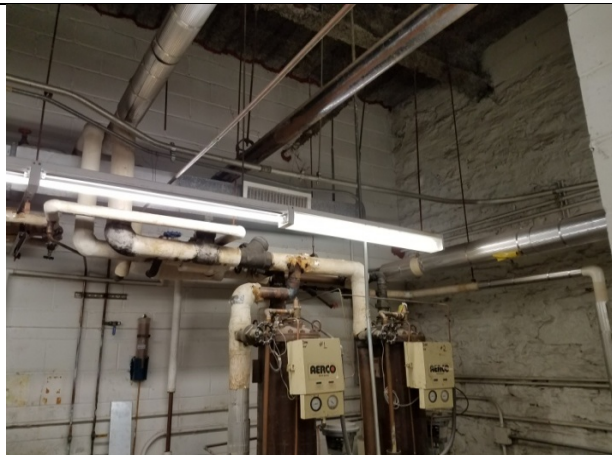
Photo P3-Existing Domestic HW Heaters
