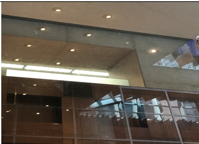
Photo M21-Supply Grilles in Reading Room
