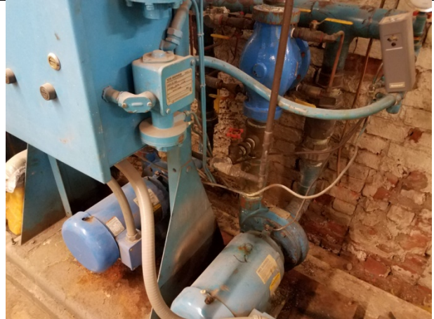
Photo P2-Existing Domestic Water Pumps
