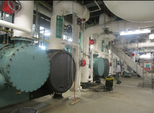
Photo M1-Central Chilled Water Plant
