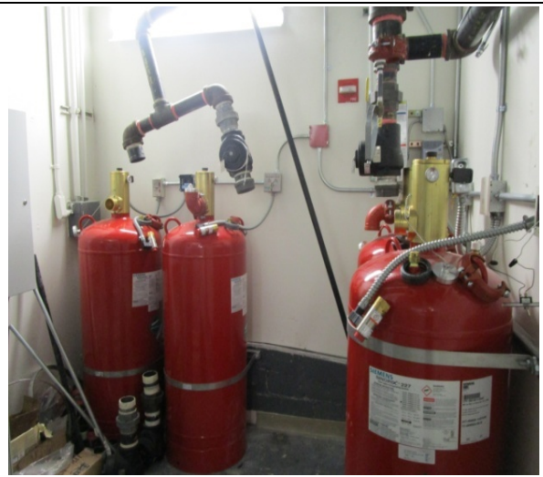
Photo FP4-Chemical Fire Suppression System
