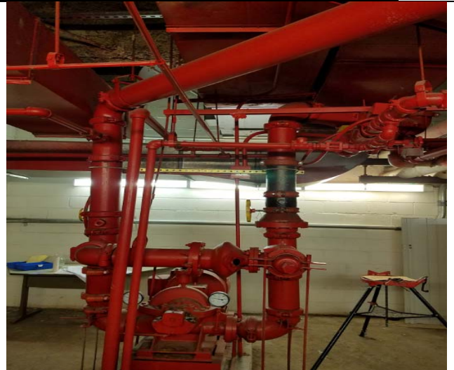
Photo FP2-Fire Pumps
