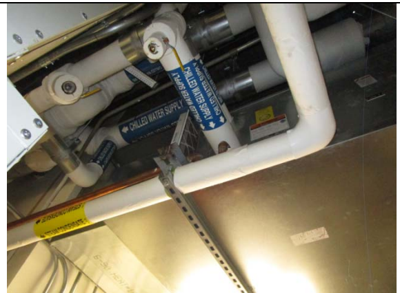
Photo M10- AHU-L-4
