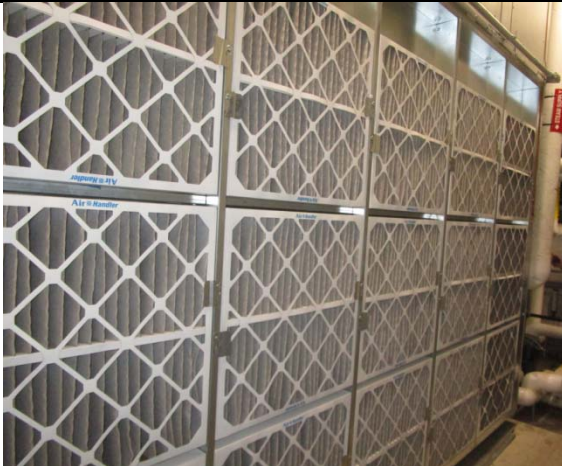
Photo M13- AHU-L-3
