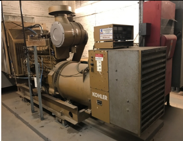
Photo E1-Emergency Diesel Generator
