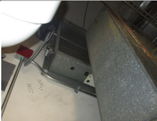
Photo M15-Smoke Purge Exhaust
