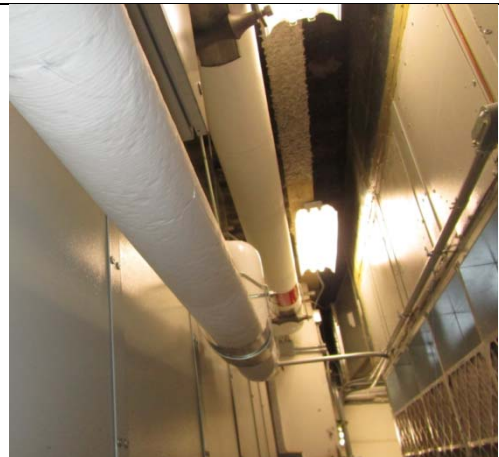
Photo M12- AHU-L-2
