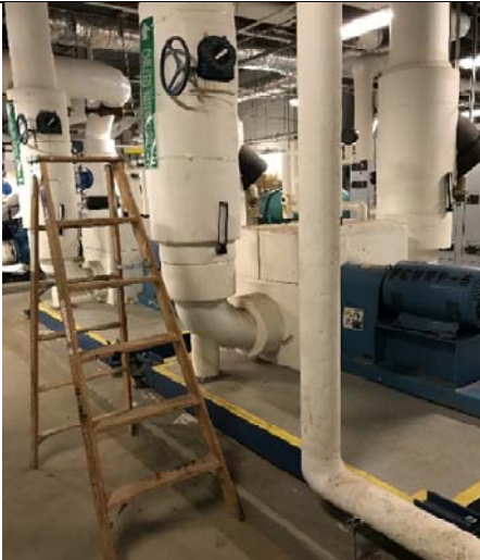
Photo M3-Primary Chilled Water Pumps
