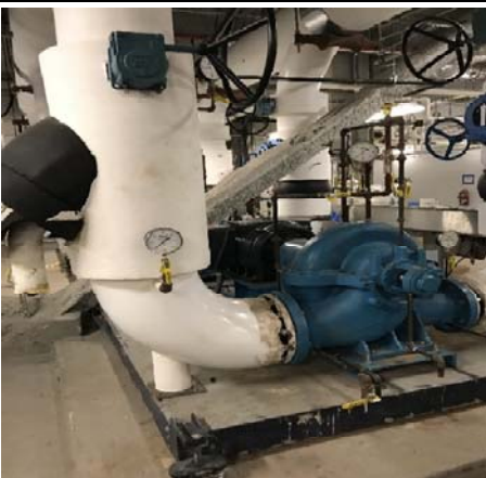
Photo M5-Condenser Water Pumps
