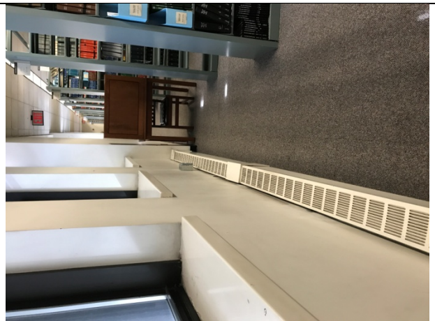
Photo M22 – Existing Fin Tube Radiators
