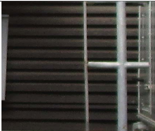
Photo M11- AHU External Louver
