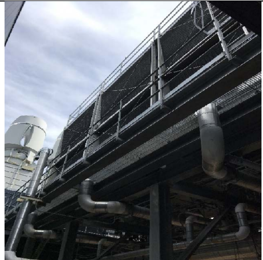
Photo M4-Cooling Tower
