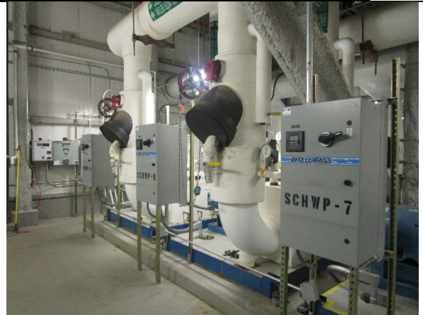
Photo M2-Secondary Chilled Water Pumps
