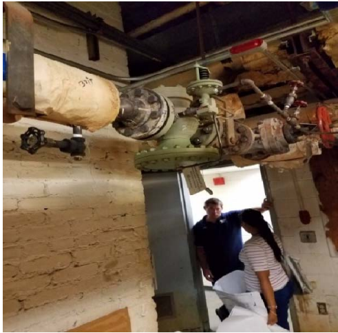
Photo M7- Steam Meter Room
