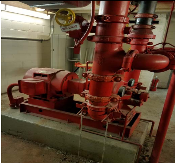
Photo FP1-Fire Pumps
