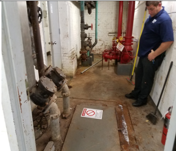
Photo FP3-Incoming Fire Service Assembly
