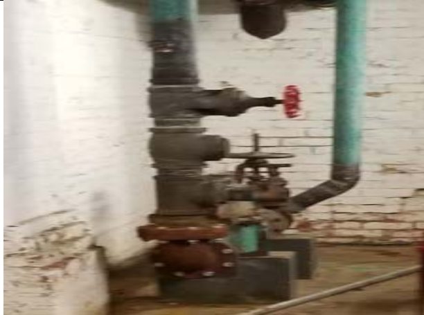
Photo P1-Incoming Domestic Water Service Assembly
